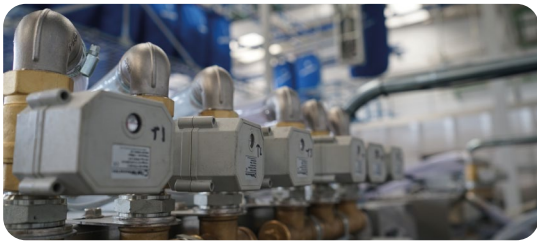
1" solenoid valves from tanks to washing machines and from pumps to tanks.
